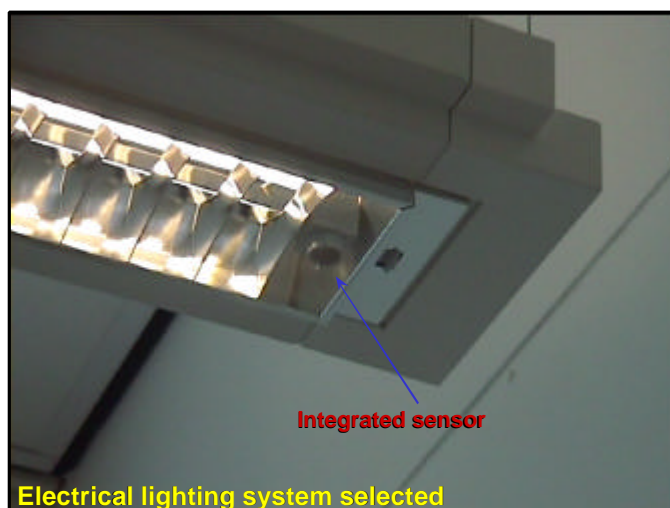
Figure 62: Electrical lighting system with integrated sensor and control.
